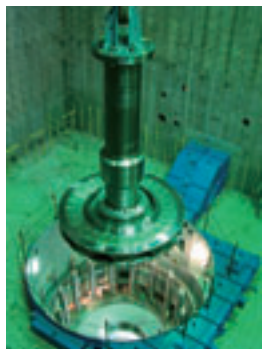
Installation of the pump turbine runner for Unit No. 2 at the Tokyo Electric Power Company's Kannagawa Power Plant
