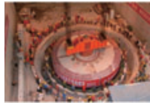
Installation of a generator rotor for the Shexigou Power Plant in China
