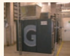
This compressor system reduces electricity consumption by 100 MWh annually.
