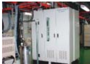
PFC gas scrubber
