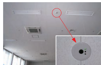
③ Energy-saving lighting system
