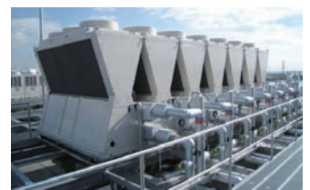
⑤ High-efficiency chillers
